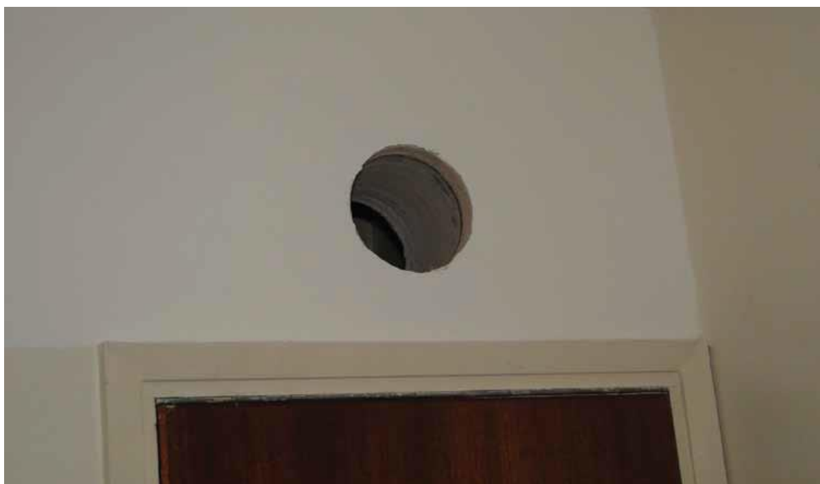
Figure 10 breach of fire-resisting enclosure
